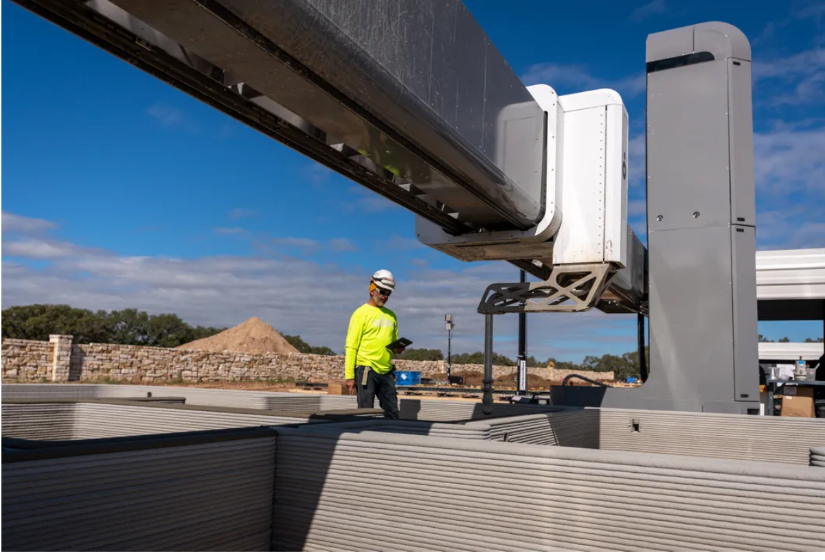
Exterior and interior walls for each 3D printed home in Icon’s 100-house project in Austin, Texas, were completed in two weeks. Lennar/Icon
