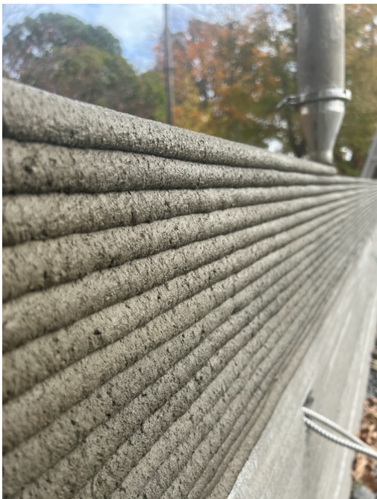
Alquist 3D is a construction firm that buys or leases printers. So far, the company has only printed straight exterior walls. Alquist 3D
